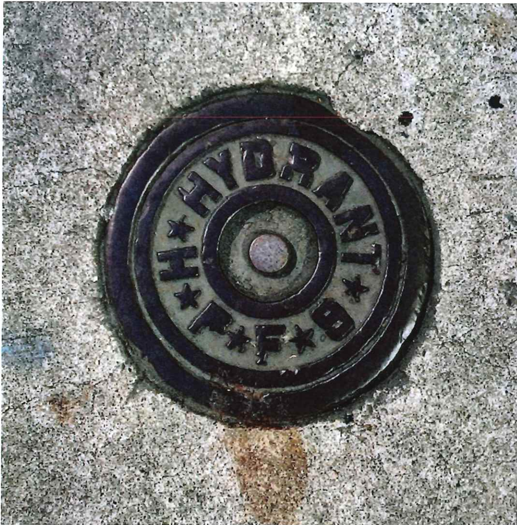
High-Pressure Hydrant Shutoff Gate Valve Cover
